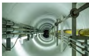
Low pressure pipelines
