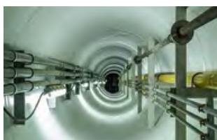
Low pressure pipelines
